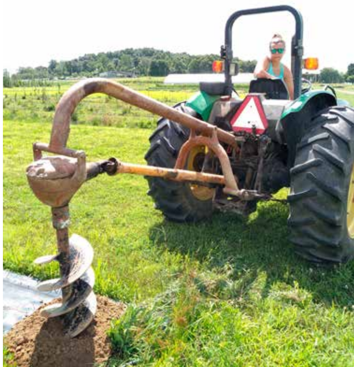
MaKayla Risner operates the tractor-mounted post hole digger during a recent trellis installation project at OSU South Centers.
